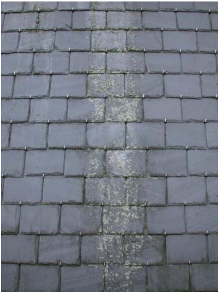
Asbestos roofing shingles appear similar to these
