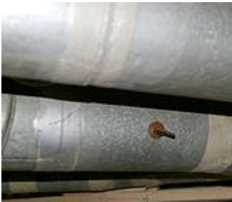
Asbestos tape on pipes
